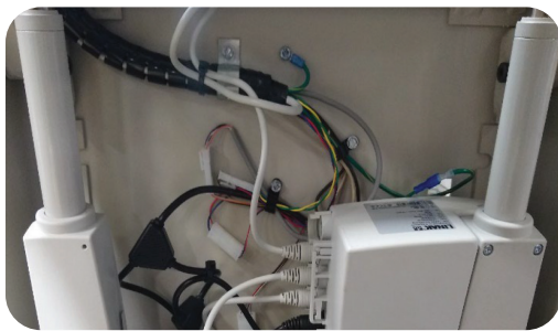
Control Box Mounted to Actuator
